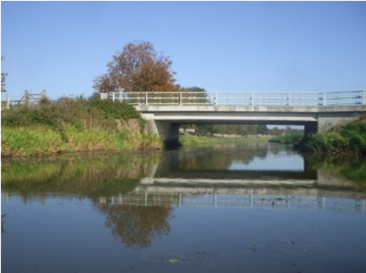
Image shows the bridge over the Royal Military Canal, Frogmore Lane, Bonnington
